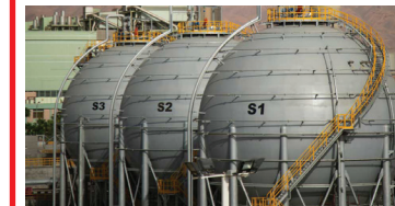
Fuel Oil Tanks
